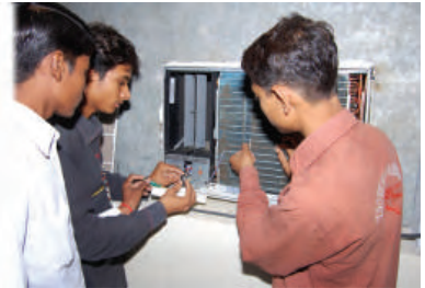
Air Conditioner Maintenance
